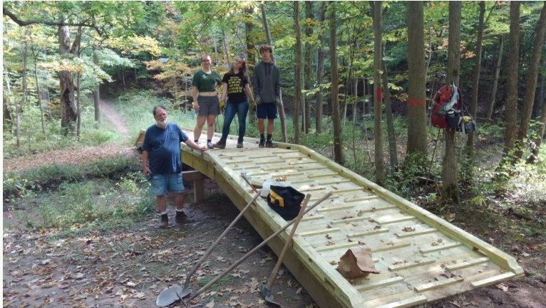
John VanBortel (far right) and some of his team putting the finishing touches on the new bridge. Photo by Chauncy Young.
